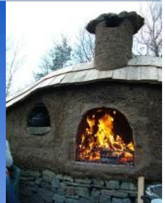
The courtyard cob fireplace at Cwmbwrla Day Centre—built by a group from the centre with Down to Earth.
